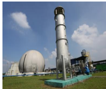
Biogas Project in RSTP Shah Alam 2
